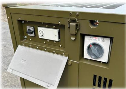
Unit Mounted Controls
